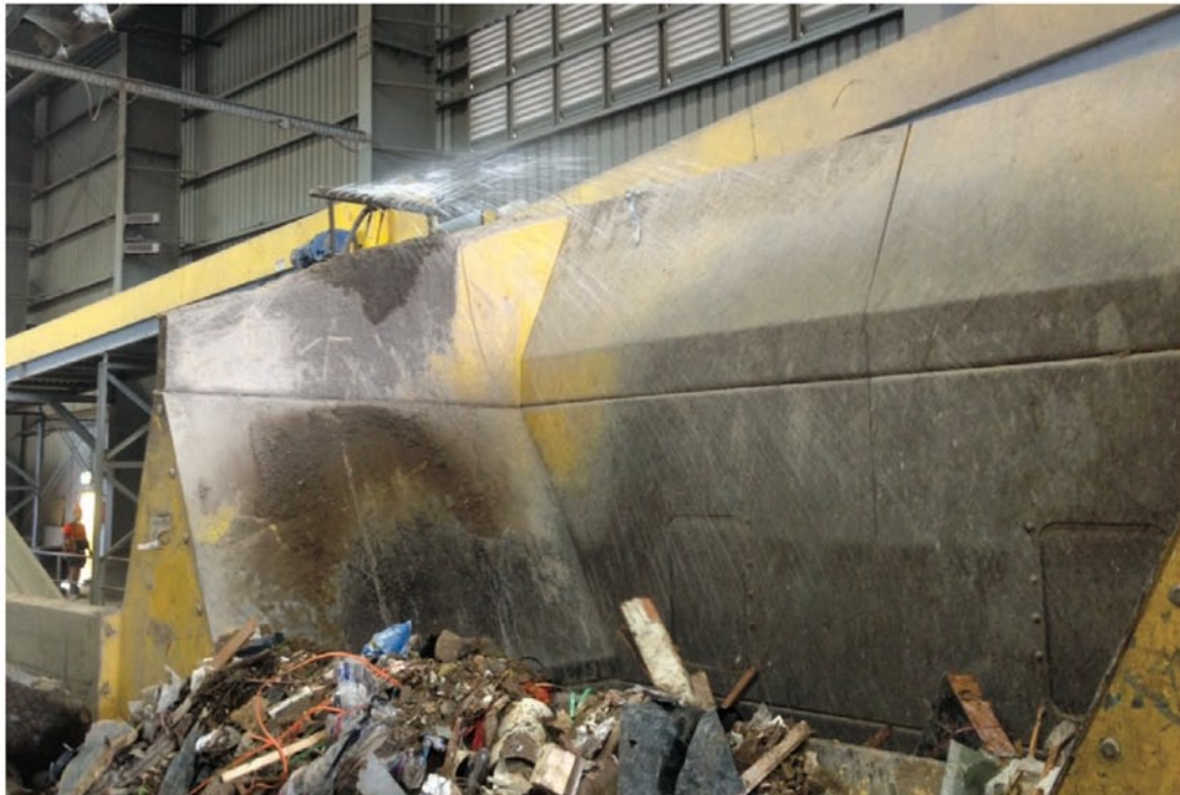
Polo BDS being sprayed onto waste material before it enters the shredder.
