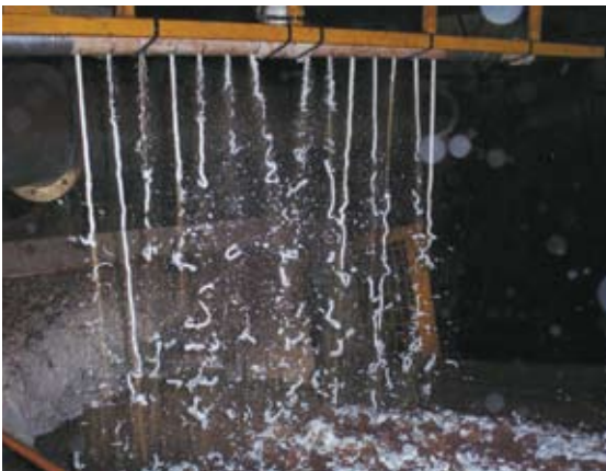
The foam suppression system in operation.
