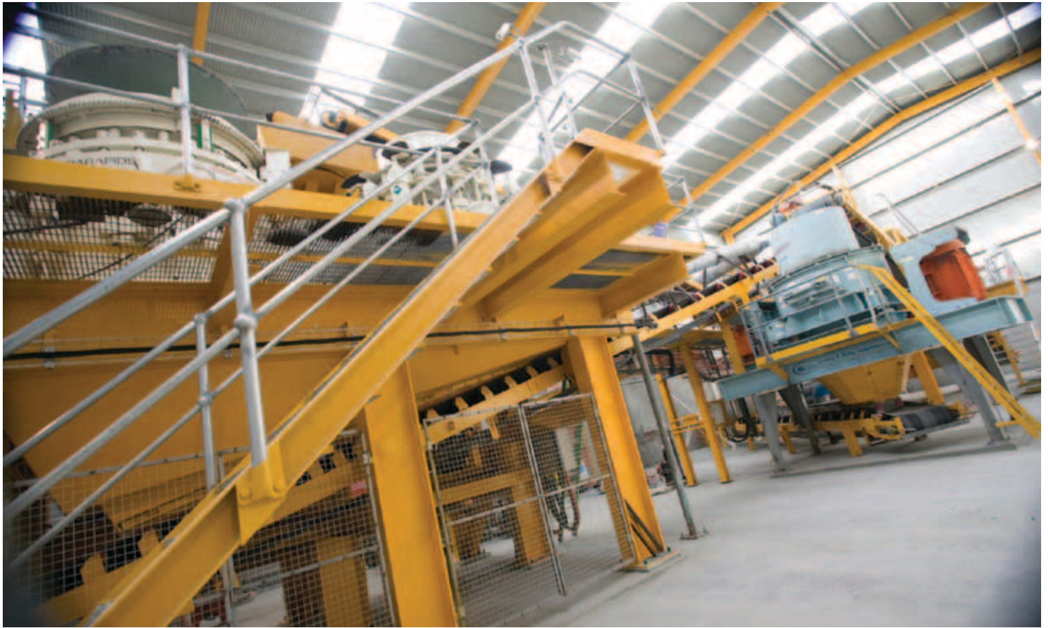
All clear: Hazell Bros' secondary and tertiary crushing and screening circuit at its Leslie Vale plant initially filled the shed with volumes of dust.
